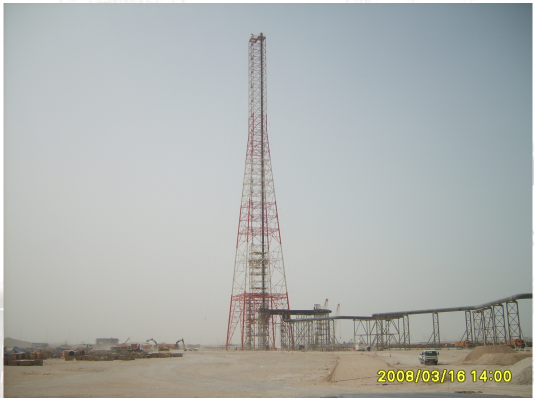
200m Height Demountable Flare - Qatar
