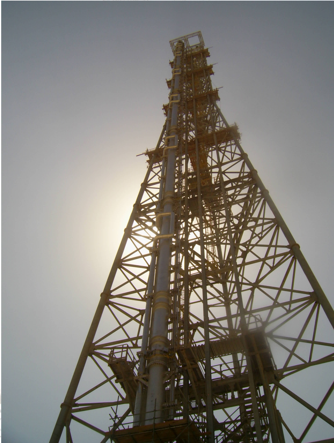
130m Height Demountable Flare - Qatar
