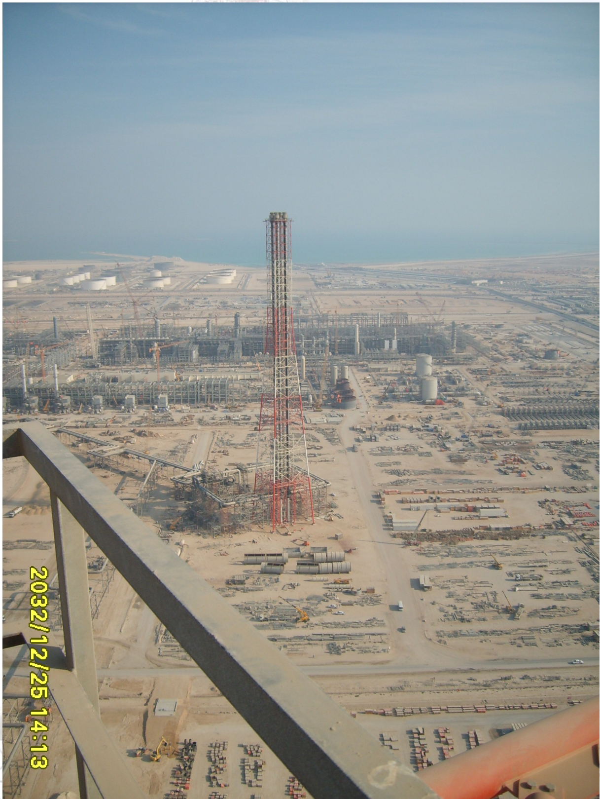
200m Height Demountable Flare – Qatar
