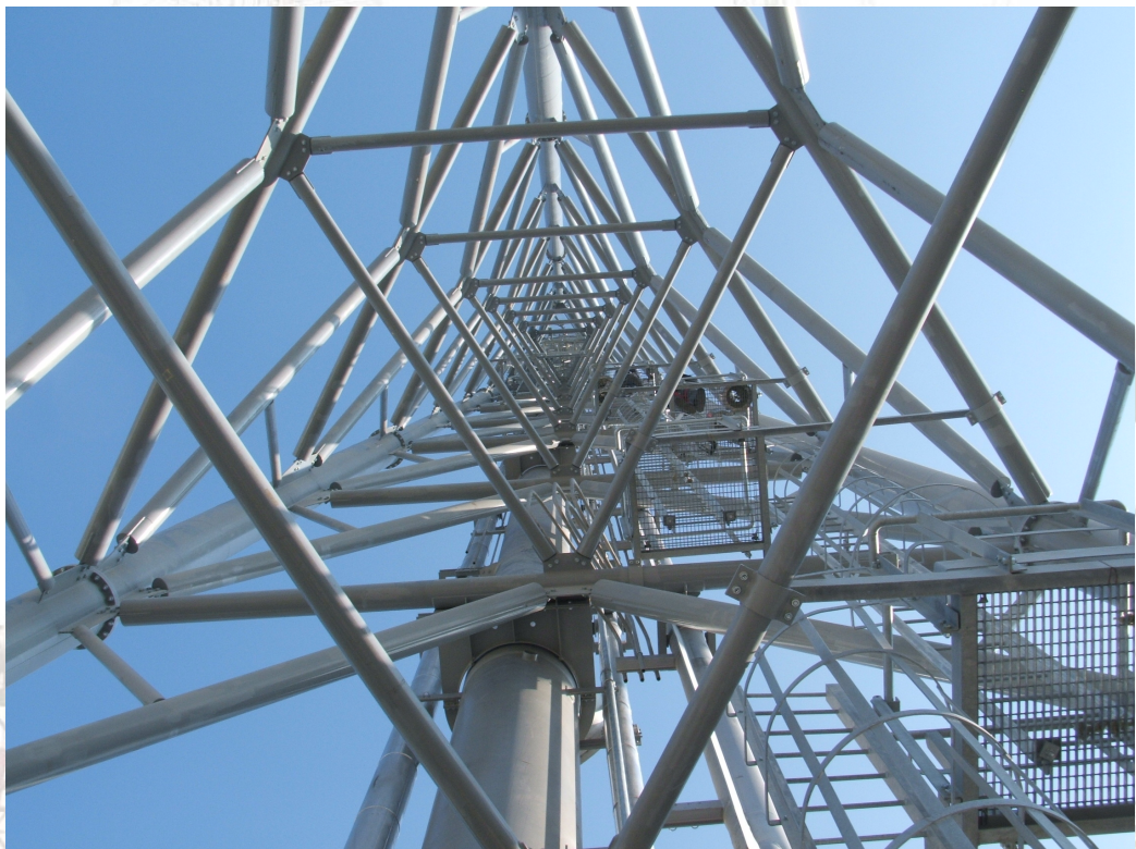
80m Height Fixed Flare - Italy
