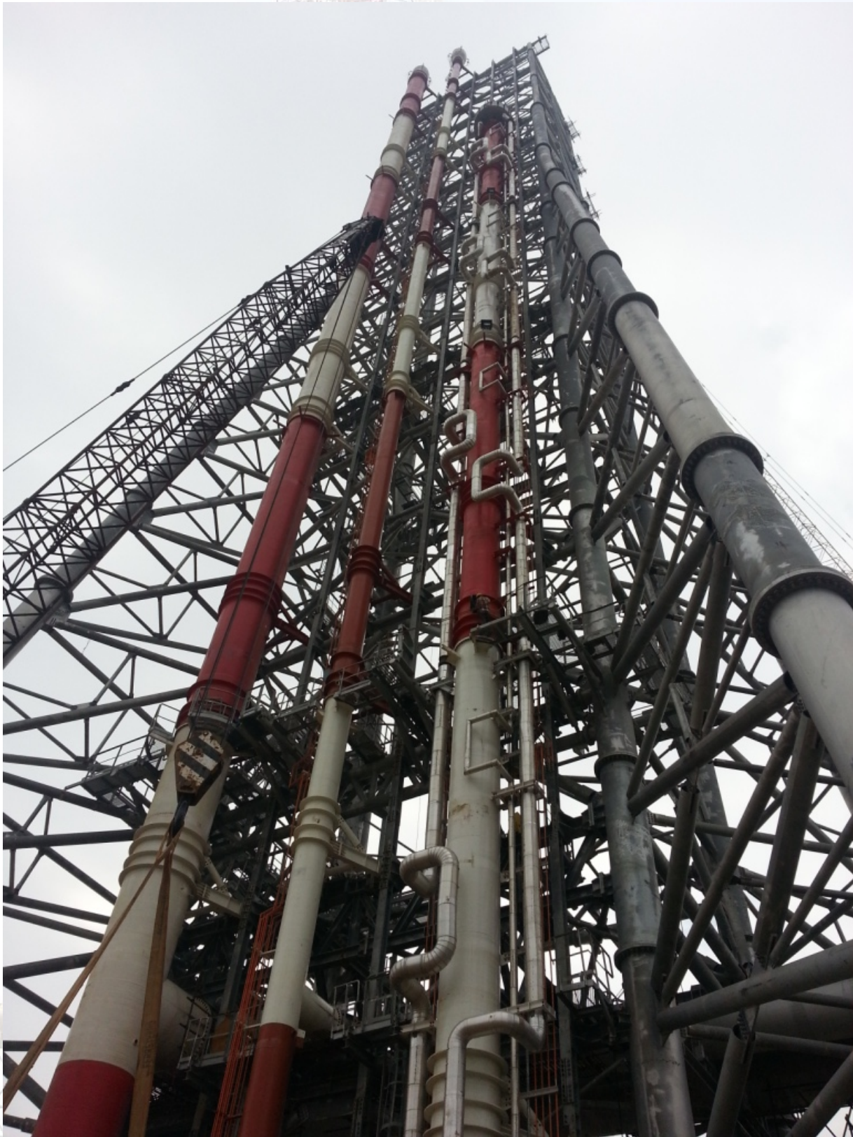
125m Height Demountable Flare – Paradip Refinery India
