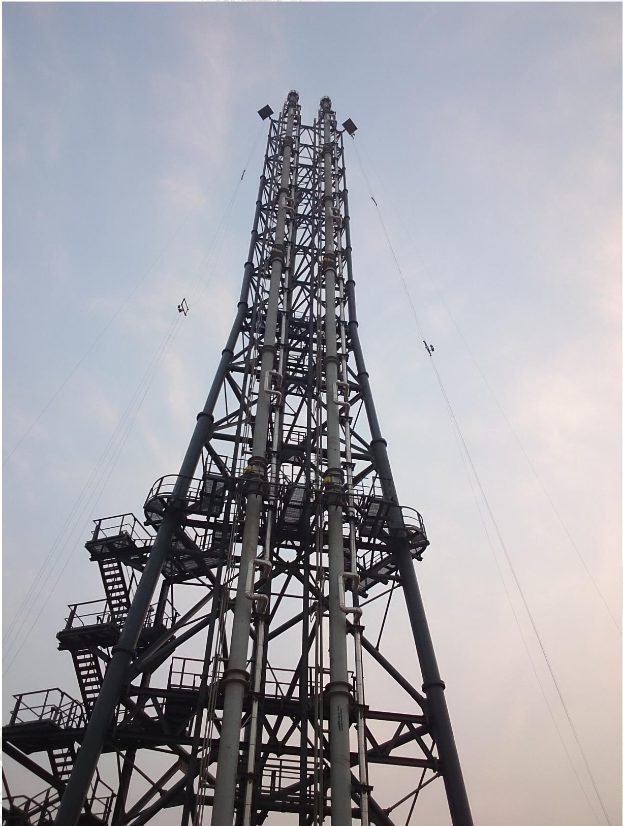
76m Height Demountable Flare – Paradip Refinery India
