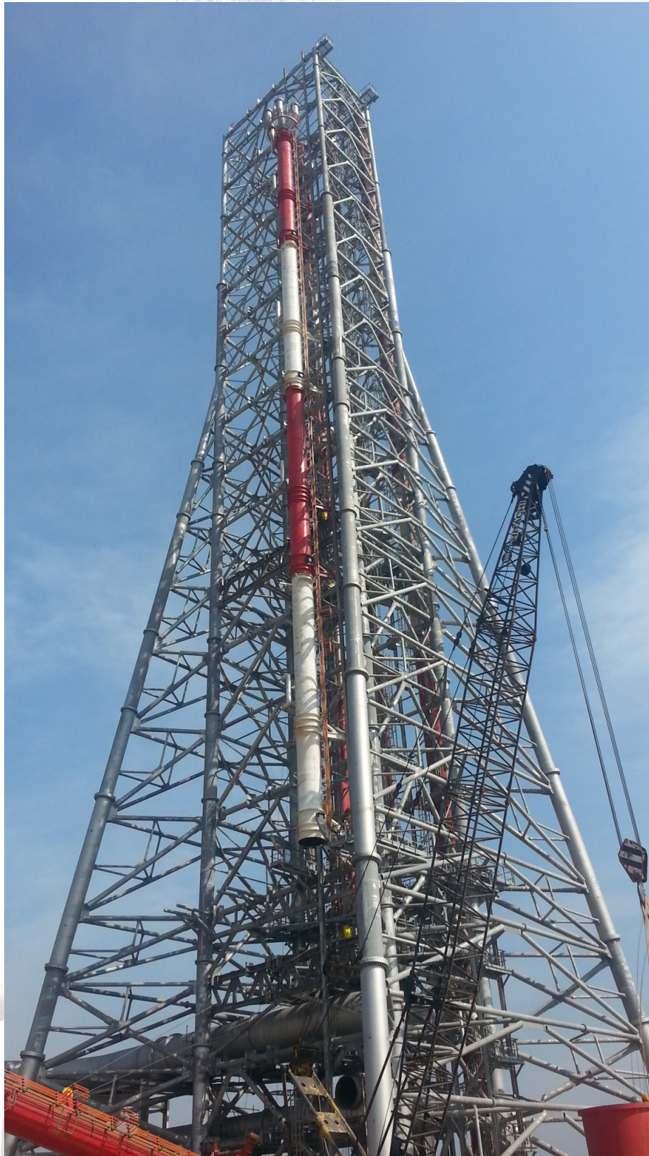
125m Height Demountable Flare – Paradip Refinery India
